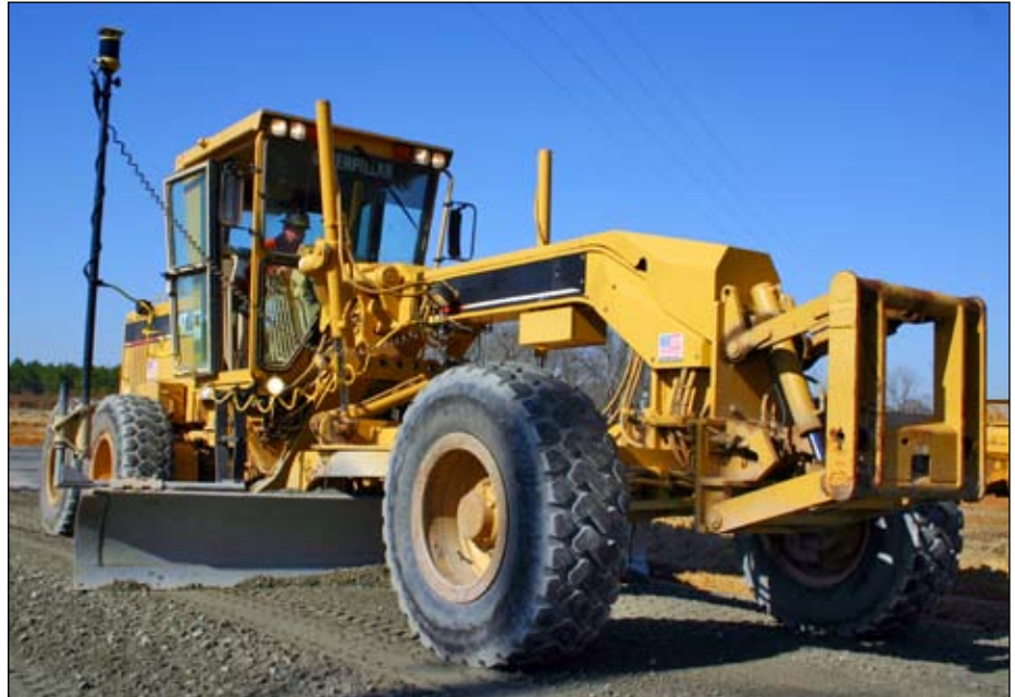
GGPC's Cat 163H motor grader finishes road base to a 1/4" tolerance with Millimeter GPS.
