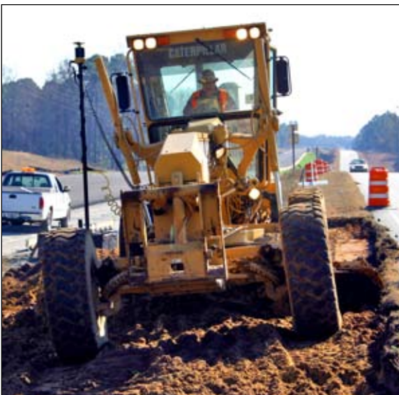
Topcon's 3D-GPS+ system enables GGPC to grade anywhere on the site without hubs and stakes.
