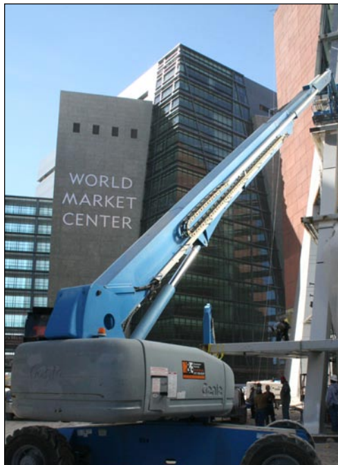
Embassy Glass drew upon the benefits of total stations as it undertook one of its most challenging wall system installations ever.
