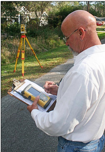
Jack Goff uses a hand-held data collector with robotic total station to plot points and survey water lines.
