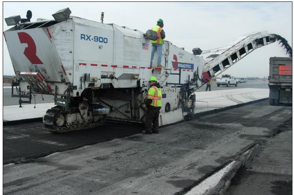
Rough-milling the existing surface to an inch and a half above finished subgrade.
