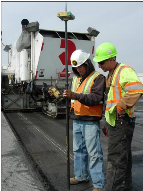
The rover allowed the exact grade to be easily verified anywhere on the airport project.
