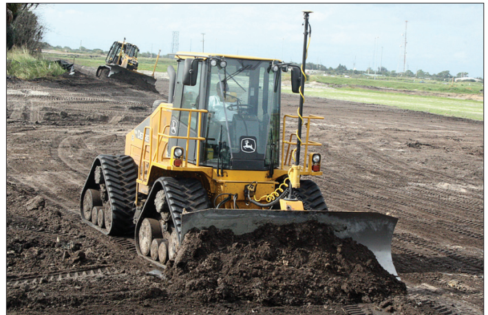
ABOVE: Fine grade - Lee Mar uses data for both soil layers loaded into its John Deere 764 HSD running Topcon's 3D-MC 2 machine control. This allows the operator to do a section of the subgrade and, when finished, simply switch offsets and grade the top layer.
