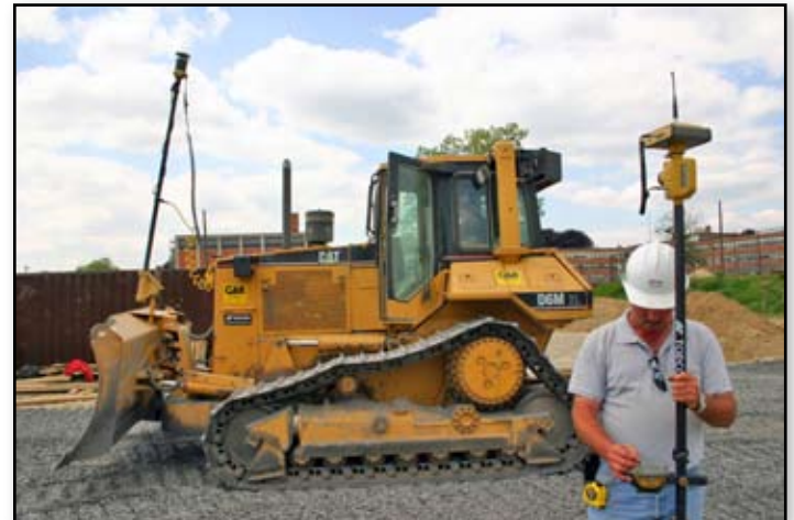
Nick Brothman , Site Superintendent, checks grade on the concrete track perimeter curb using a Topcon HiPer+ with mmGPS+ and an FC-100.
