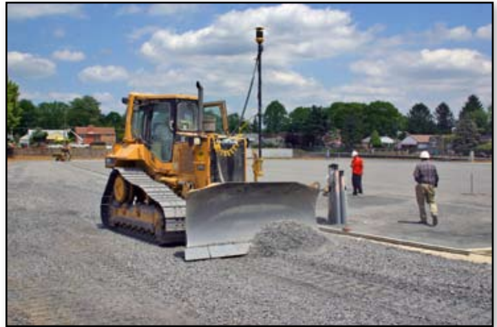
Seravalli used Topcon’s mmGPS+ with their System 53D-GPS+ equipped Cat D6M for fine grading this running track.
