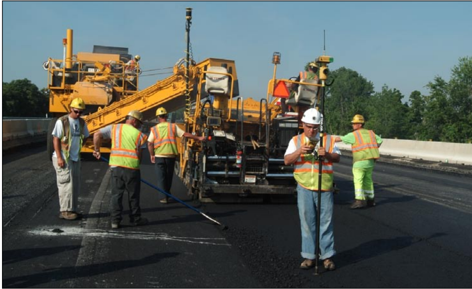
Ray Tripp, surveyor for Myers, checks the grade of the uncompacted asphalt on the Turnpike project. Paving the Turnpike was a high-production project; Allan A. Myers averaged 2,500 tons of hot mix per shift.
