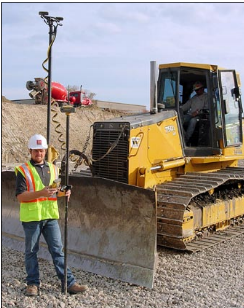
Chris Aspegren, project manager for Berger Excavating, checks location footings using a Topcon HiPer Lite+ rover unit and an FC-200 Pocket 3D field monitor.
